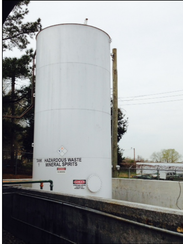
Photo # 13: RCRA Permitted Used Parts Washer Solvent Storage Tank (S02) inside Parts Washer Solvent Tank Farm. Photo taken 4/10/14.
