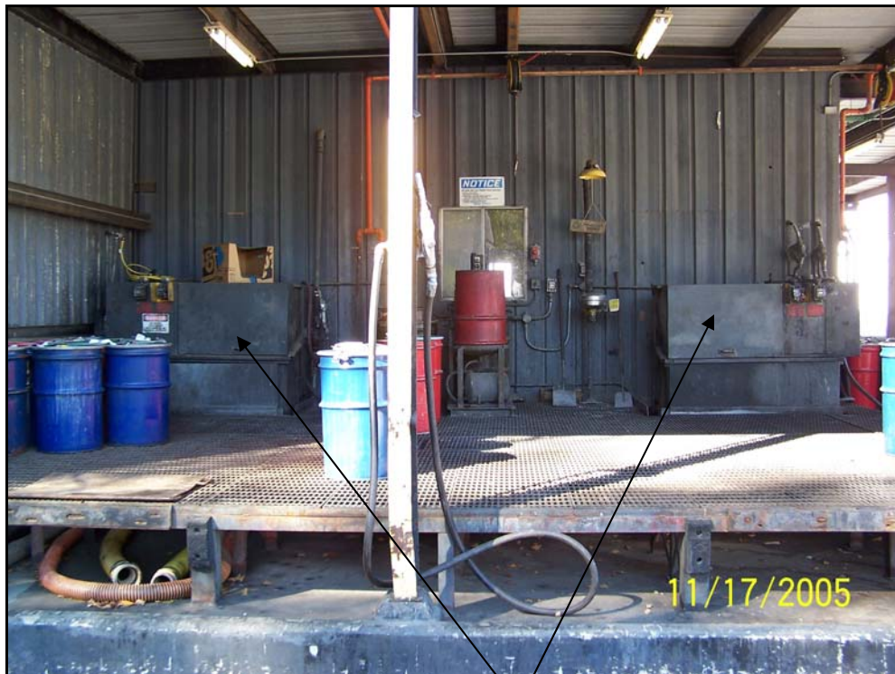
Photo # 10: Drum Washer/Dumpster Units (X99) located at Return and Fill Area.
