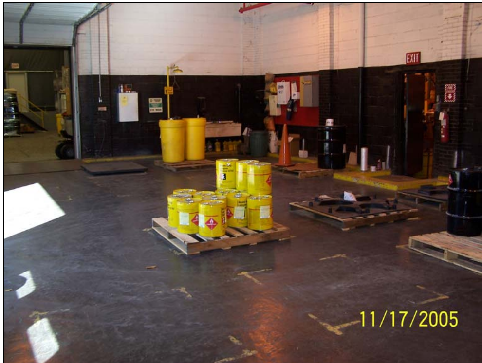
Photo # 8: RCRA permitted Class 1B Flammable Container Storage Area (S01) looking north.
