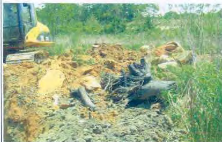
Photo E: Large stumps and trash in TP-11.
