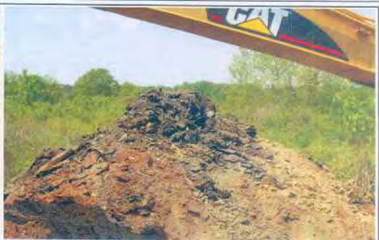
Photo H: Shingles and trash in TP-14.
