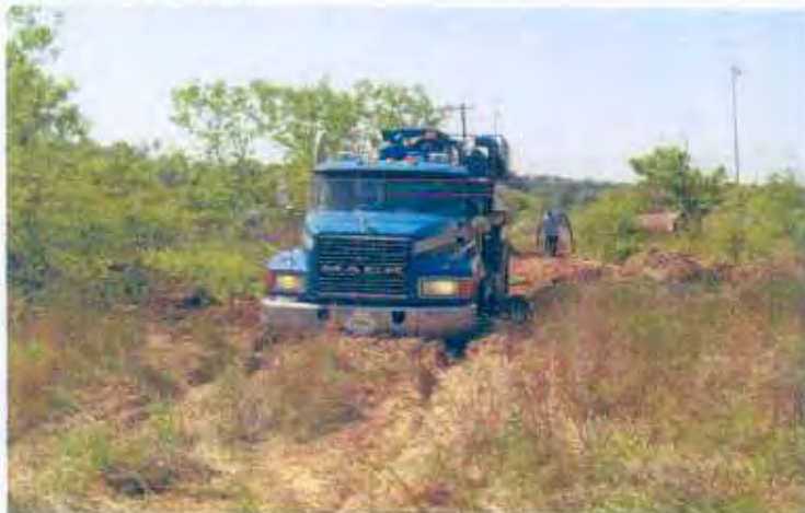
Photo Q: Haz-mat Tanker onsite to vacuum gas and water from tank.
