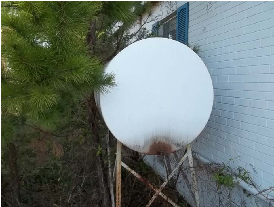
Photograph 8: Heating oil AST located on Tract 2.
