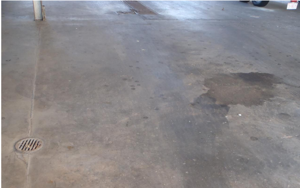
Photo 7 –Floor drain and stains inside northeast building.
