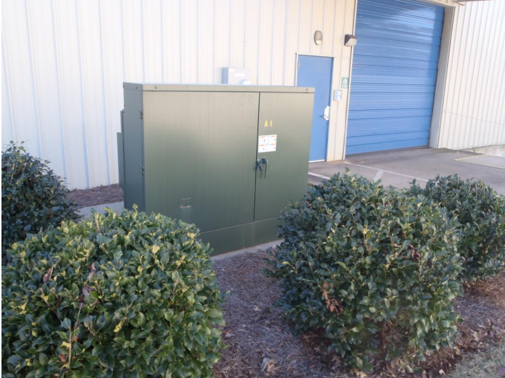
Photo 5 – One of two pad-mounted transformers located on the project site.
