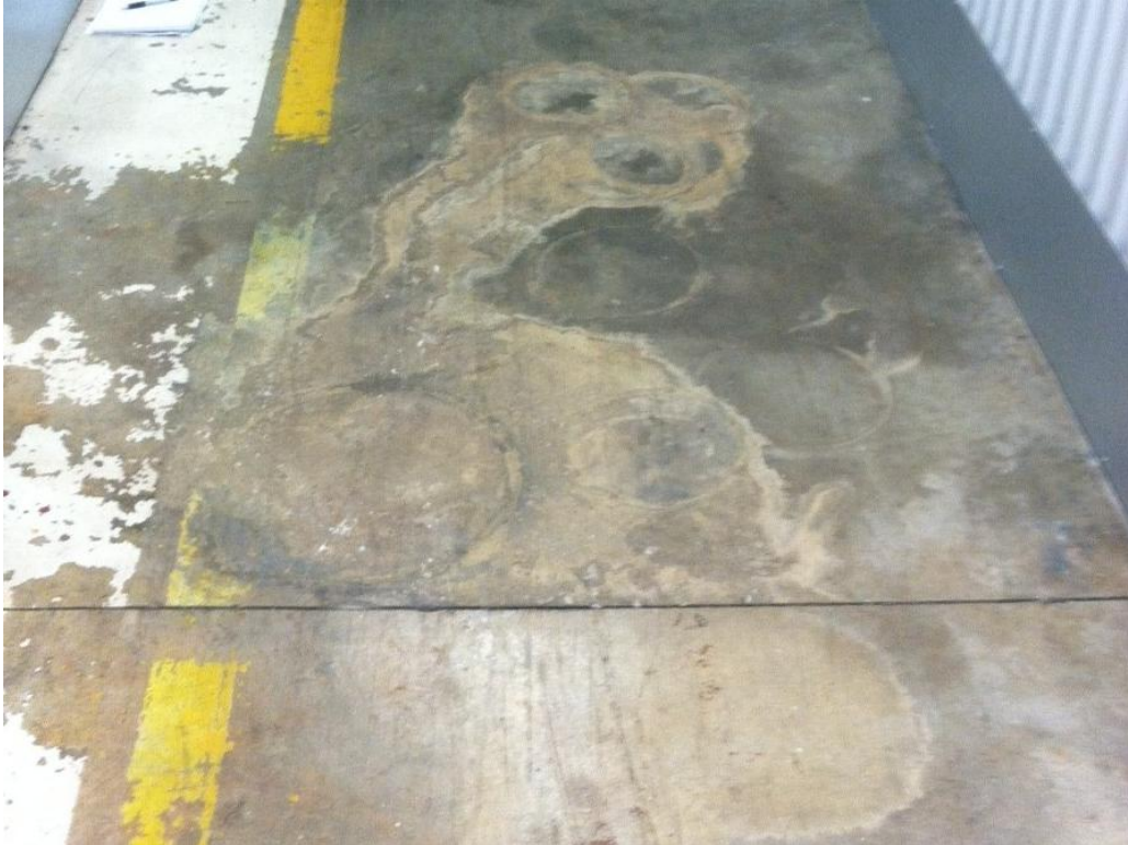
Photo 3 – Stains and indentions on the floor of the southeast building.
