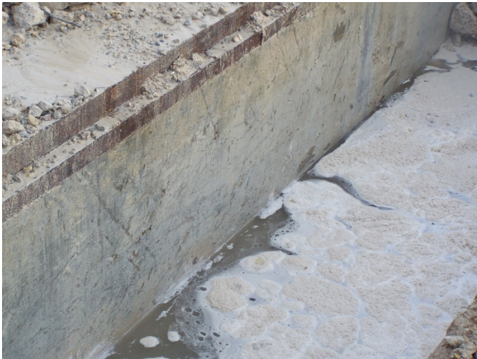
Photograph #7- SWMU #11- Spray Line Sump Walls
