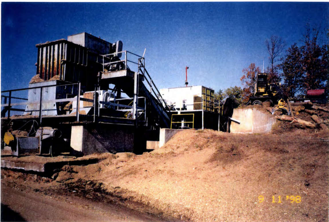
Yardwaste and Pallet Processing Unit, looking northwest (Horizontal Salvage Hog and Hammer Mill).
